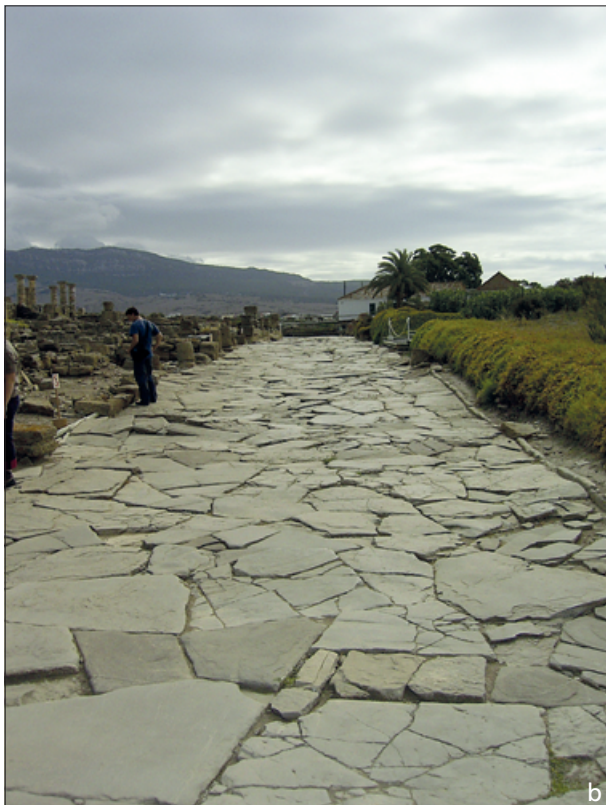
Fig. 15 a Italica (Santiponce). Tiled pavement of the cardo maximus in front of the Casa de la Exedra. Note the folding due to the creep towards the NW (red arrow indicates slide). – b Baelo Claudia (Bologna). Tiled pavement of the decumanus maximus , the deformation was interpreted as earthquake damage. – (Photos K. Reicherter).
