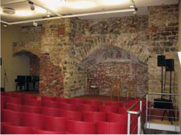
Fig. 10: The 13th century city wall in the Hungarian Cultural Centre, Treurenberg, Brussels (© MRBC-DMS).
