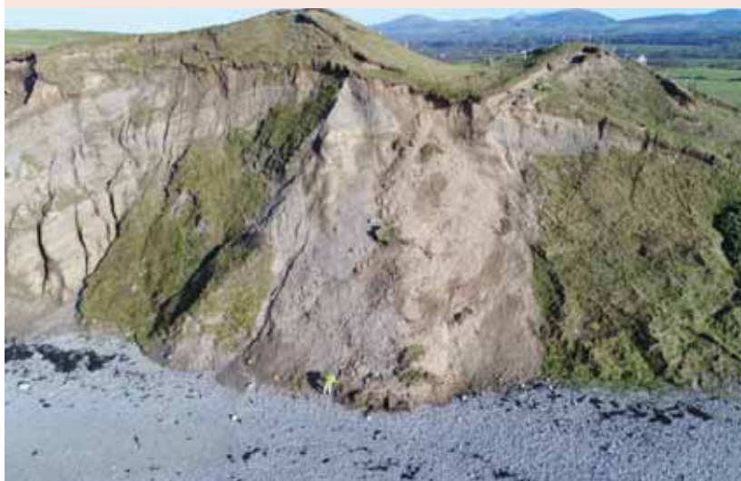
Fresh cliff collapse below the southern hillfort ditch, recorded on 14 Feb 2019, was exacerbated by intense rainfall funnelling water along the fort's ditch. Crown Copyright: CHERISH Project 2019
