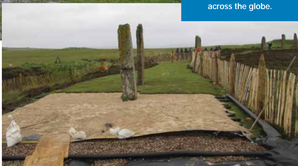
(right) Installation of engineered surfaces to improve footpath resilience at the Ring of Brodgar. Credit: Historic Environment Scotland
