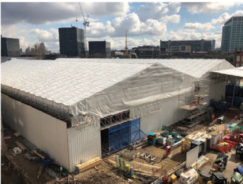
Encapsulation structure over the big dig at St James's Gardens in Euston designed by Costain Skanska JV. Credit: Caroline Raynor, Costain Skanska JV; © HS2 Ltd
