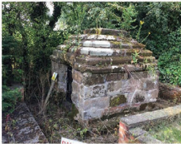
Grade 2 listed plunge bath at Manor Farm, Streechay, 18th century (monitored for cracking and water level drop). Credit: WSP; © HS2 Ltd
