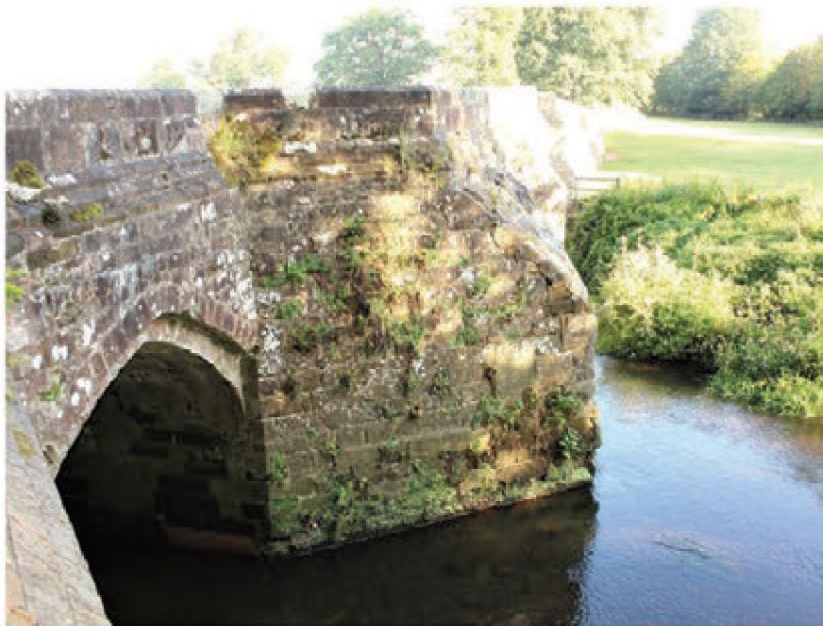
Scheduled and Grade 2* listed Stare Bridge, Stoneleigh Abbey, 15th century (monitored for cracking) Credit: WSP; © HS2 Ltd
