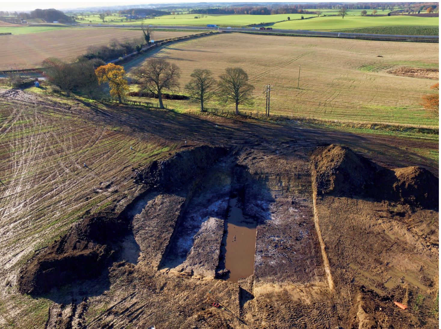
Aerial view of excavations following initial stripping and sampling works on one of the kettle holes ©Archaeological Research Services Ltd
