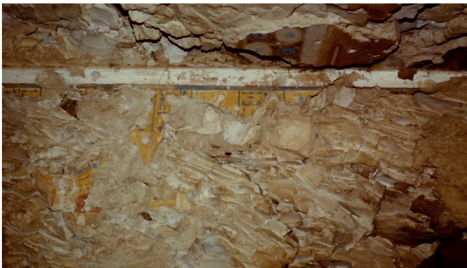
FIG. 4: Right side of the left lintel over the entrance to the passageway in TT 118.
