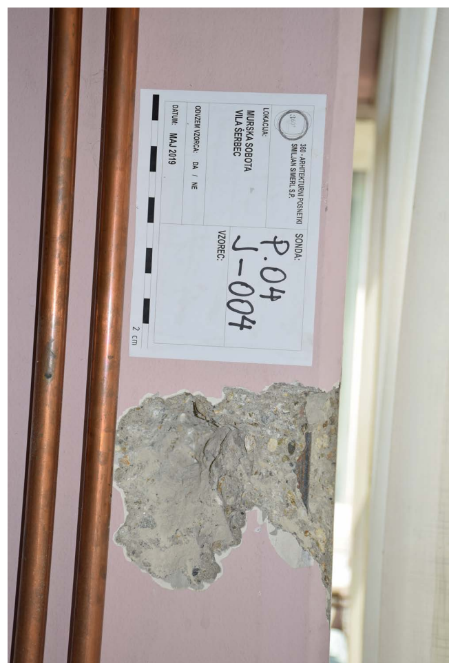
9 Research of the structure on the pier: determining the preservation of the primary piloti under the secondary layer of concrete. Photo: Smiljan Simerl, 2019
