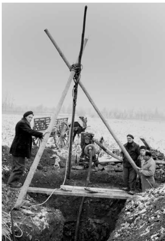
Fig. 10. Vix. The block and tackle – a triangular structure made of timber beams designed to support the hoist for lifting the crater – is being installed by the Roblin company (Marcel Roblin is on the right, wearing a beret and glasses; his son, Roger Roblin, also wearing a beret, is on the left). A horse (who went by the name of Mouton) harnessed to a cart can be seen in the background.
