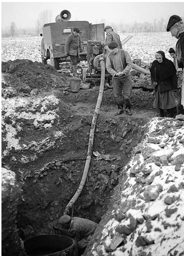
Fig. 9. Vix. Maurice Moisson, at the bottom of the hole containing the crater, is busy installing the water pump.
