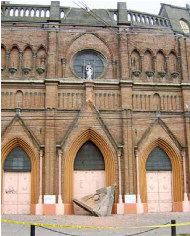
Corazon de Maria, damaged church
