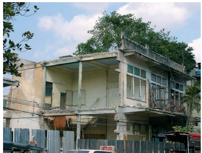
Half-demolished house in Wang Li community
