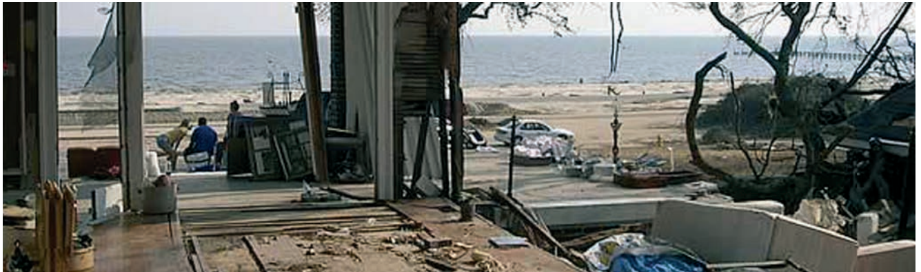
House on the Mississippi Coast, damaged by Hurricane Katrina
