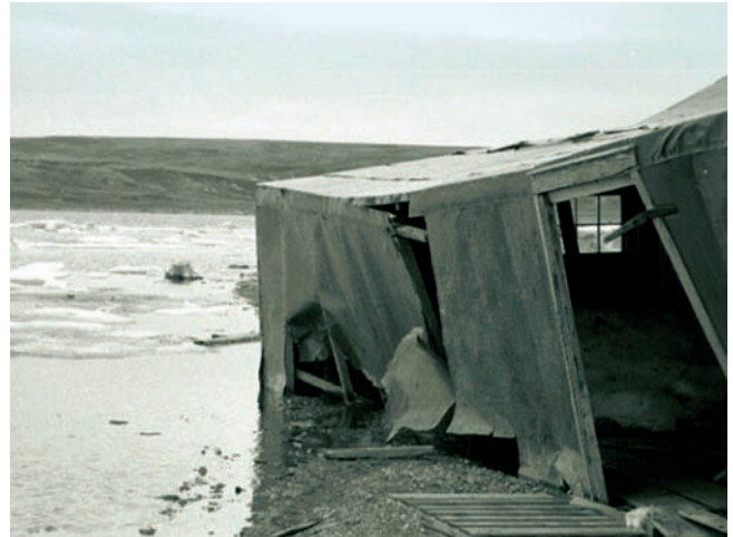
June, 2001 - the NW&TCo Store shed addition after being crushed by sea ice the previous fall (Credit: Government of Yukon Territory)
