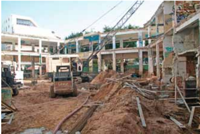
Building on Dizengoff Square, beginning of demolition work on the courtyard side (photo: B. Furrer)
