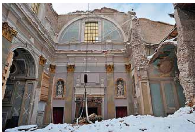
L'Aquila, the heavily damaged church of Santa Maria Paganica
