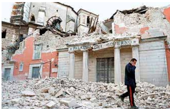
The Palazzo del Governo after the earthquake
