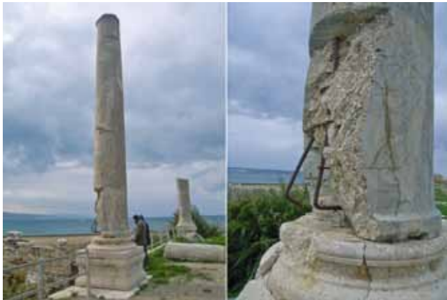
Exposed steel reinforcements from previous reconstructions. Columns could be struck by lightning during storms and thus be destroyed further
