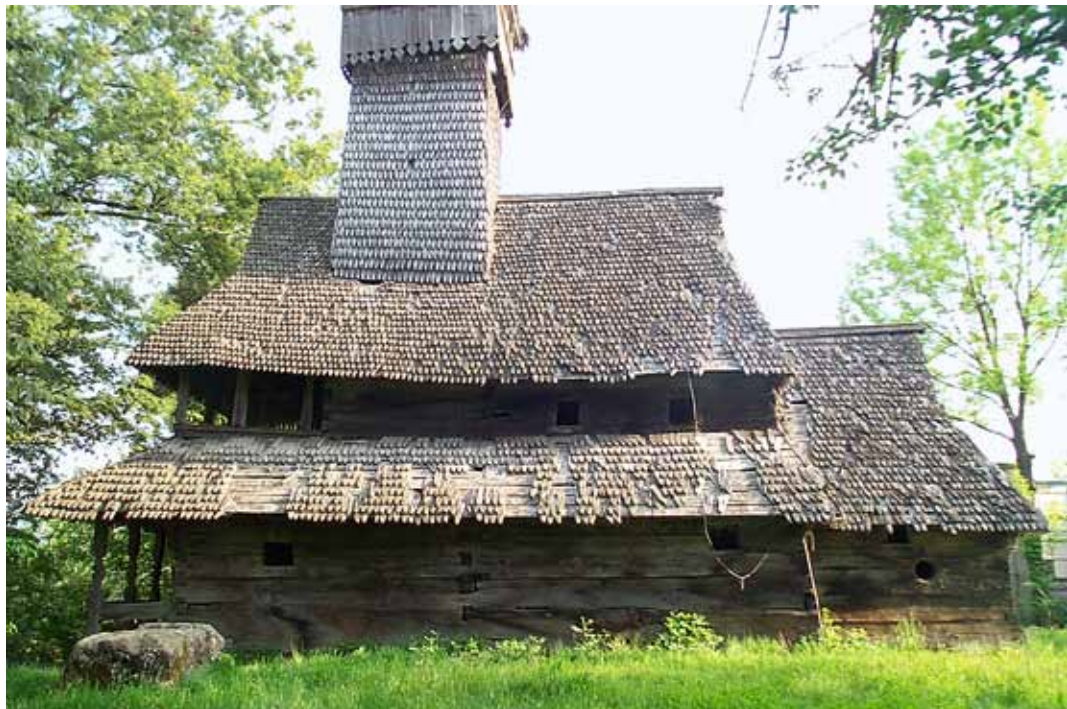
Roof damage on the south side of the church in Kolodne (photo: A. Kutnyi)
