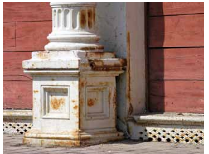
Galveston, cast iron damage
