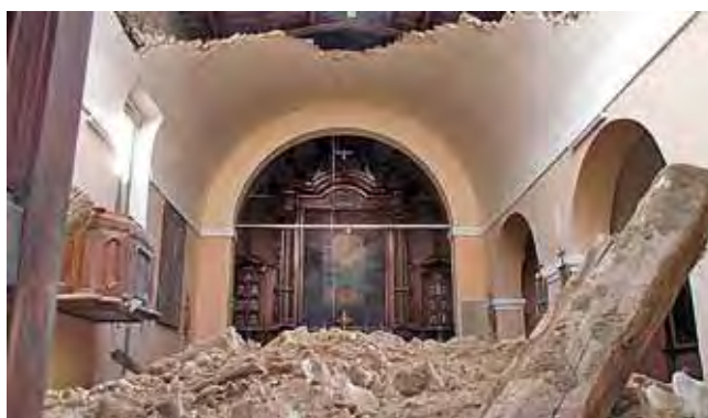
Urbino, Marche, Capuchin monastery dating from the 16th century: the collapse of the timber roof truss caused the masonry vault underneath to collapse as well.
