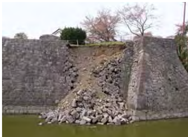
Collapsed masonry walls of Komine Castle
