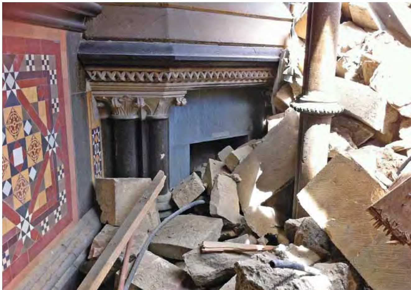
Canterbury Provincial Council Buildings, damaged interior (photo: Jenny May)
