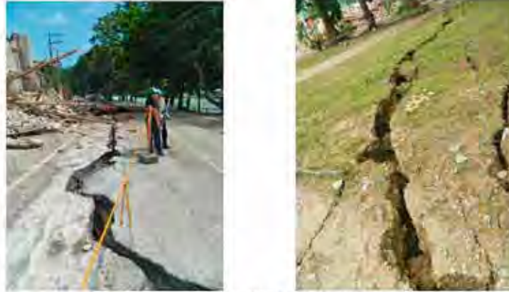
Ground cracks Loboc church (L); Maribojoc church(R)
