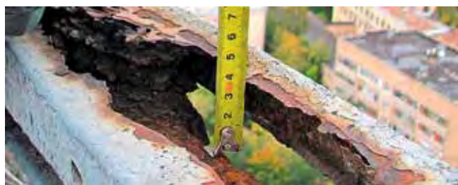
Detail of the tower's lattice work showing crevice corrosion
