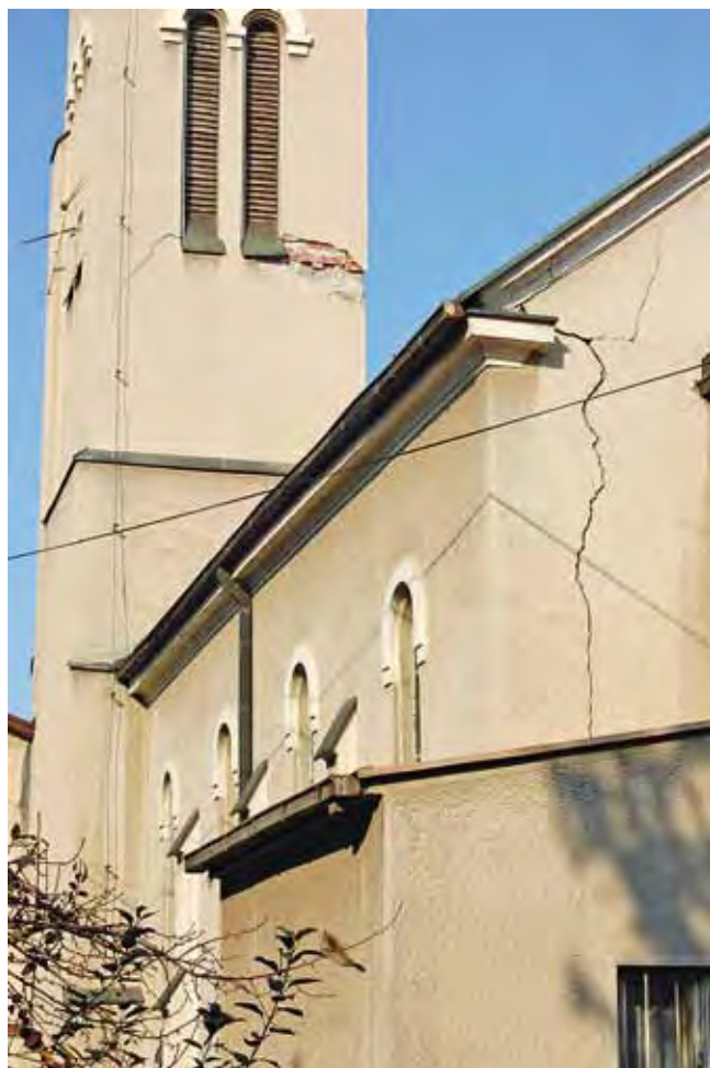
St. Michael's Church, cracks on the tower and on the church walls
