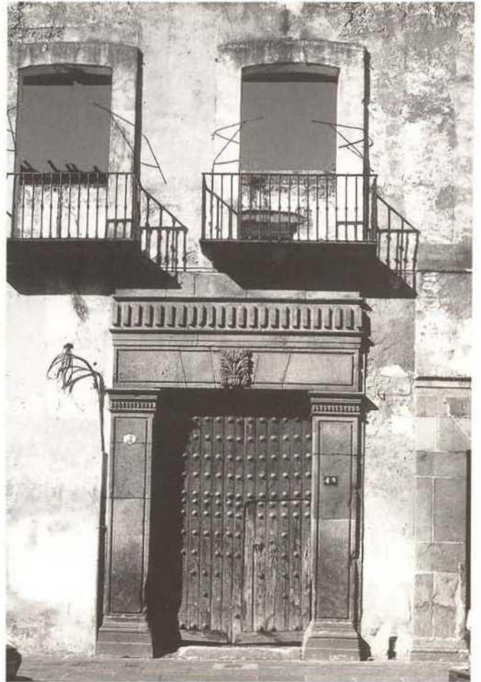
Puebla, house in the process of serious decay
