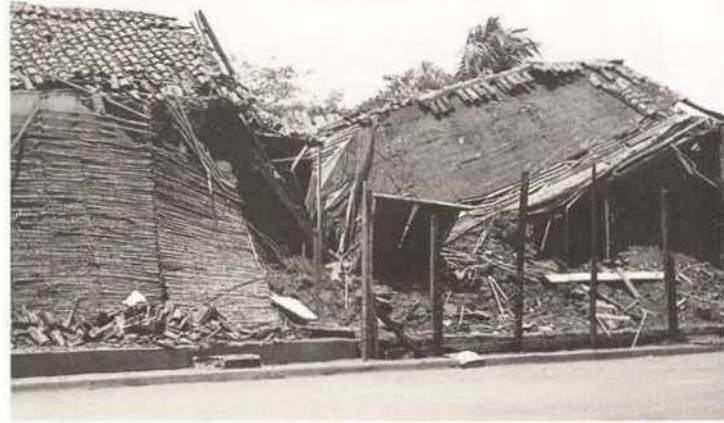
Collapsed adobe house in the historic centre of Masaya, damages caused by the earthquake of July 7, 2000
