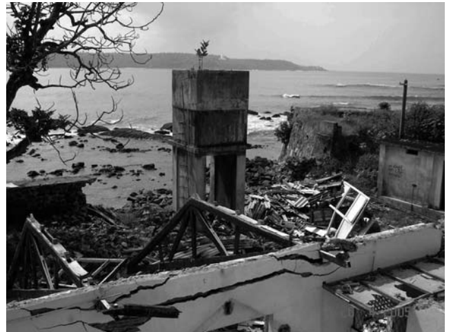
Fig. 4 Damage to rampart wall near Akersloot Bastion in Galle Fort
