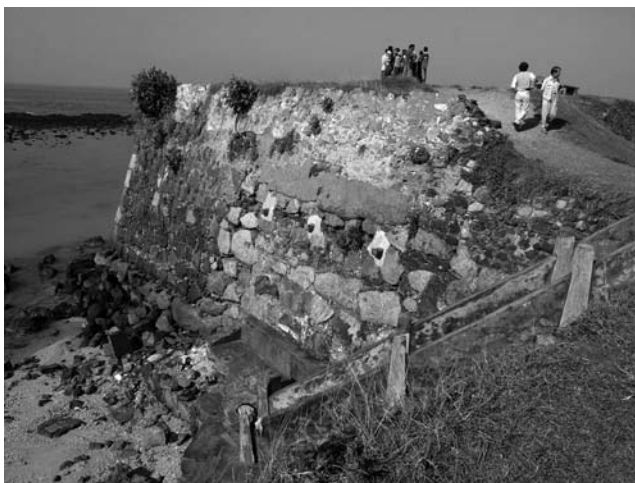
Fig. 5 Damage to rampart wall near Akersloot Bastion in Galle Fort
