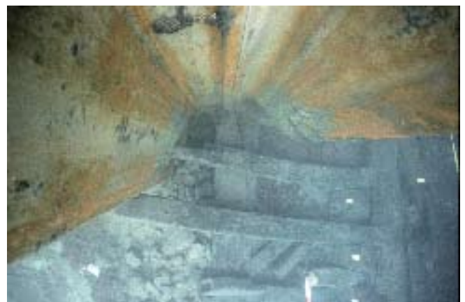
Figure 1: View of the point where the metallic bulkhead of the pier cuts the structure of the boat without damaging the rest of the architecture
