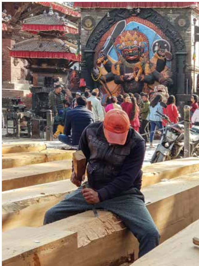
Fig. 2a: Carpenter working on a timber post for the reconstruction of Kathamandap, with the Kal-Bhairab statue in the background (© ICOMOS Nepal/Kai Weise)
