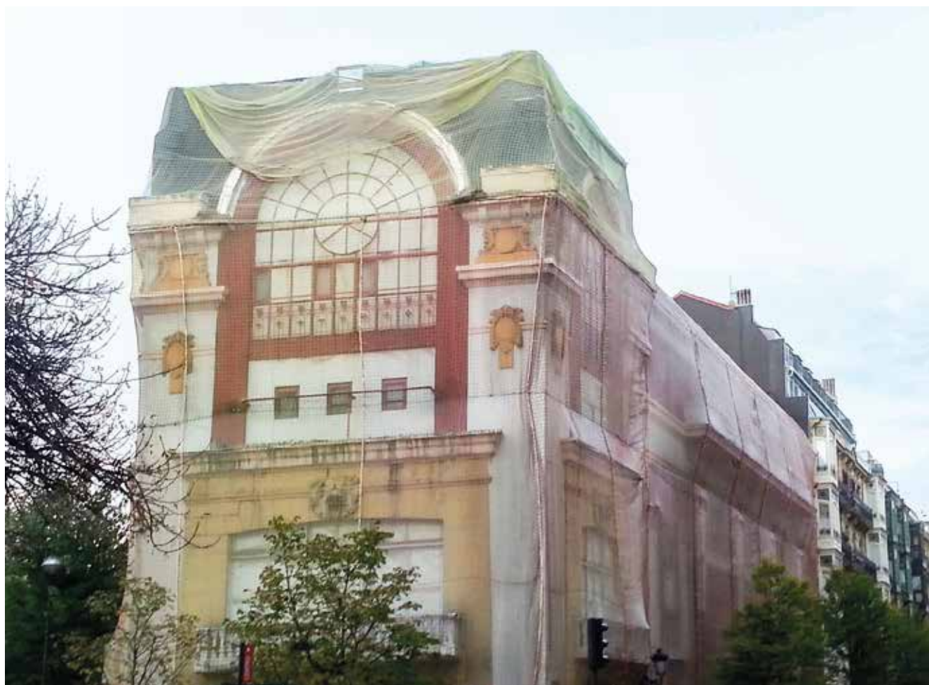
Fig. 2: Condition of the Palacio after the demolition of the dome in 2015 (© archive of author)
