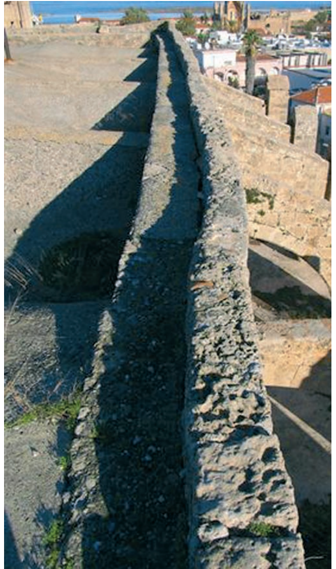
Fig. 18 An unstable wall – Saint Peter and Paul
