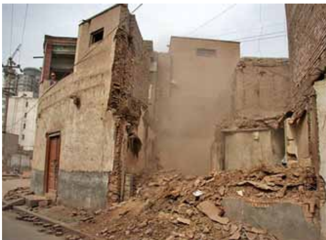
Partially destroyed building in the Old City (source: www.rferl.org)
