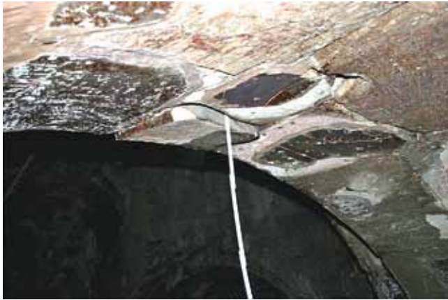
Sioni Church, cap stone in the vault of the south conch: the stone has sunk 30 mm (photo: Barthel & Maus)
