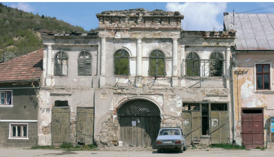
Dilapidated façade in the centre of Roşia Montana (Photo: M.Pz.)
