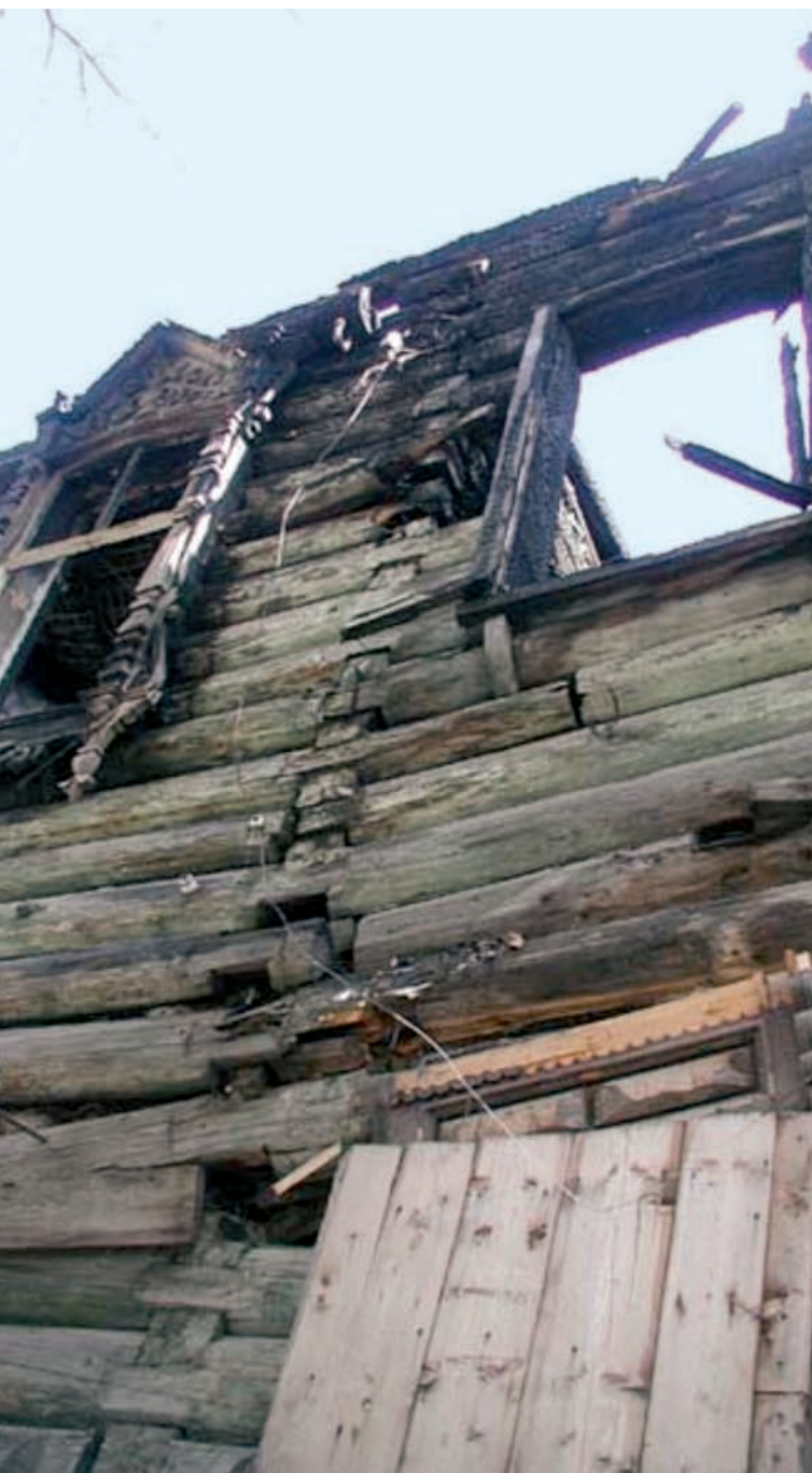
Semi-destroyed historic wooden house in Tomsk, Siberia (Photo: Jean-Luc Bruandet)
