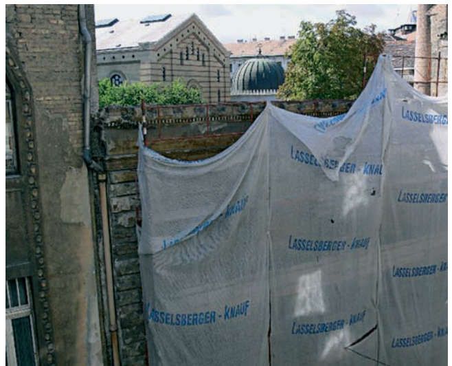
Demolition of historic buildings in Síp Street, close to the Synagogue in Dohány Street.
