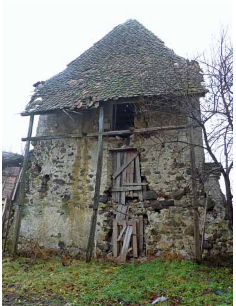
Drăușeni (Draas), fortified tower showing lack of maintenance (photo: C. Machat)
