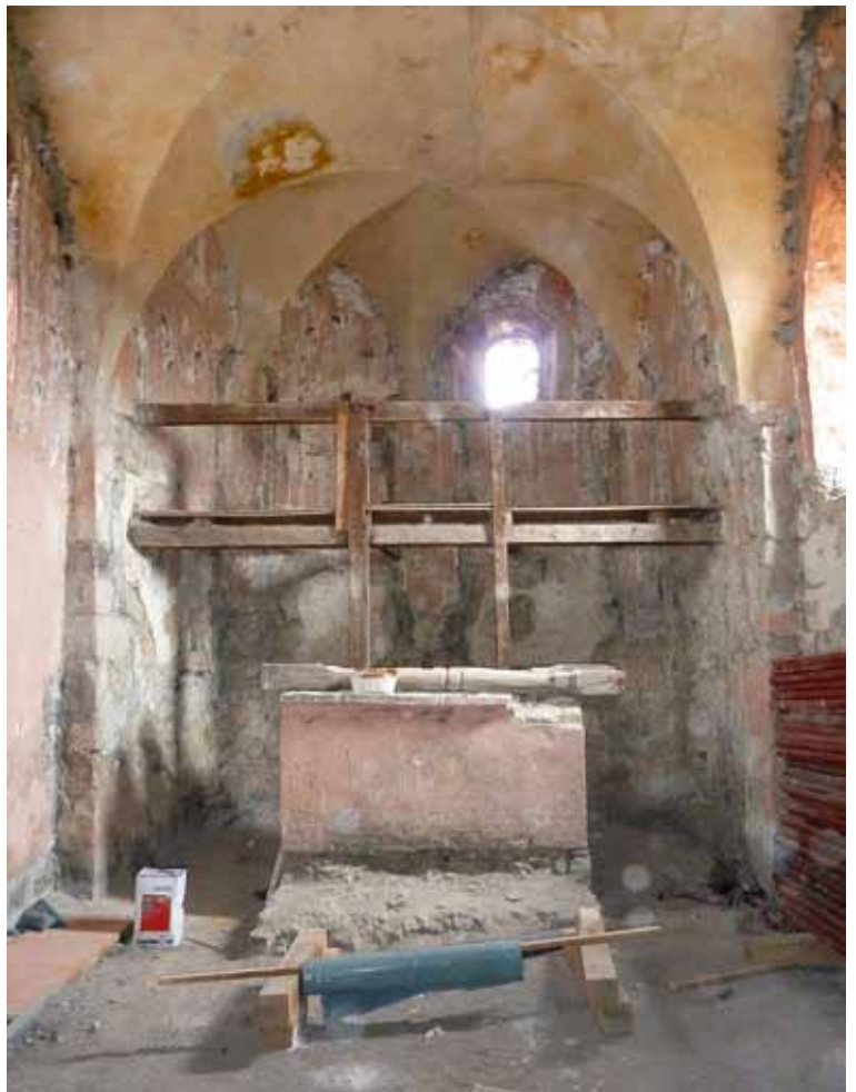
Drăușeni (Draas), church interior in a state of neglect (photo: C. Machat)
