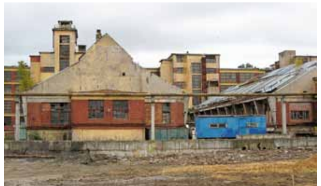
Krasnoje Znamja Textile Factory, two dyeing workshops in the courtyard, 2008 (photo: A. Zalivako)
