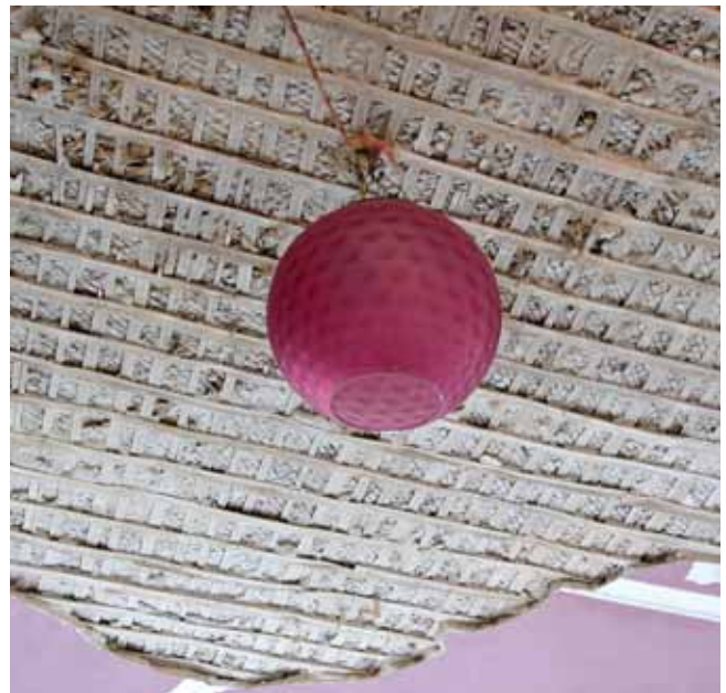
Melnikov House and Studio, ceiling damages, 2009 (photo: K. Block).
