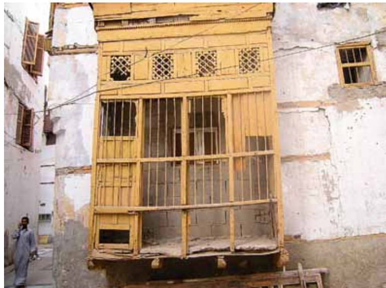
Jeddah, views of the historic centre, merchant mansions (photos: E. M. Deubzer, 2008)
