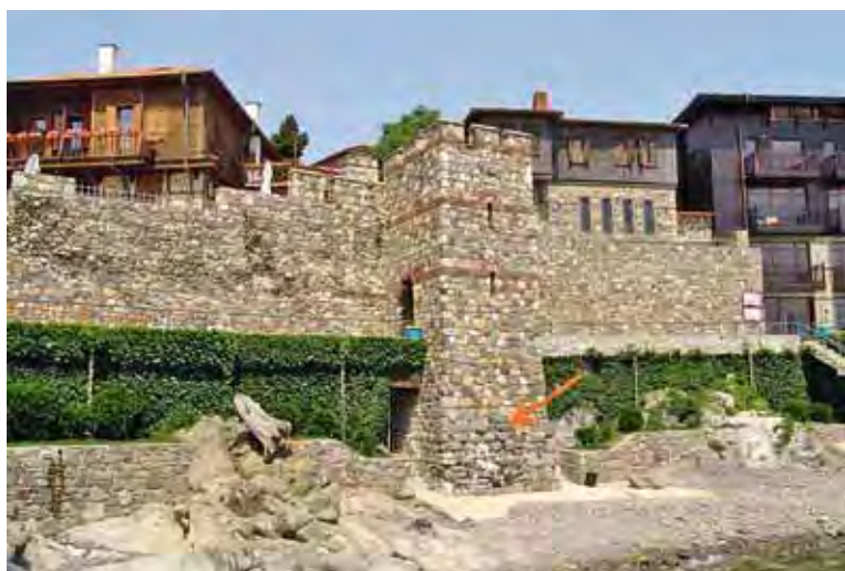
Sozopol, the original part of the tower is preserved in its base only, whereas the rest is new masonry
