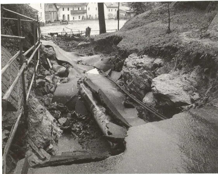
Ceský Krumlov, the condition of the access road under the Plášťový Bridge after the water falling off
