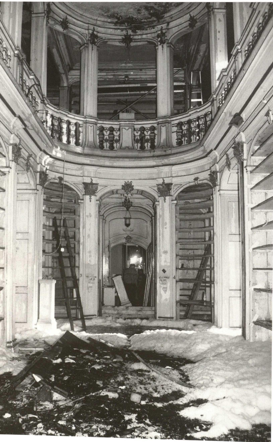
The cleared-out Rococo hall after the fire with remains of debris and foam as well as with provisional shoring (photo: J. Seifert)
