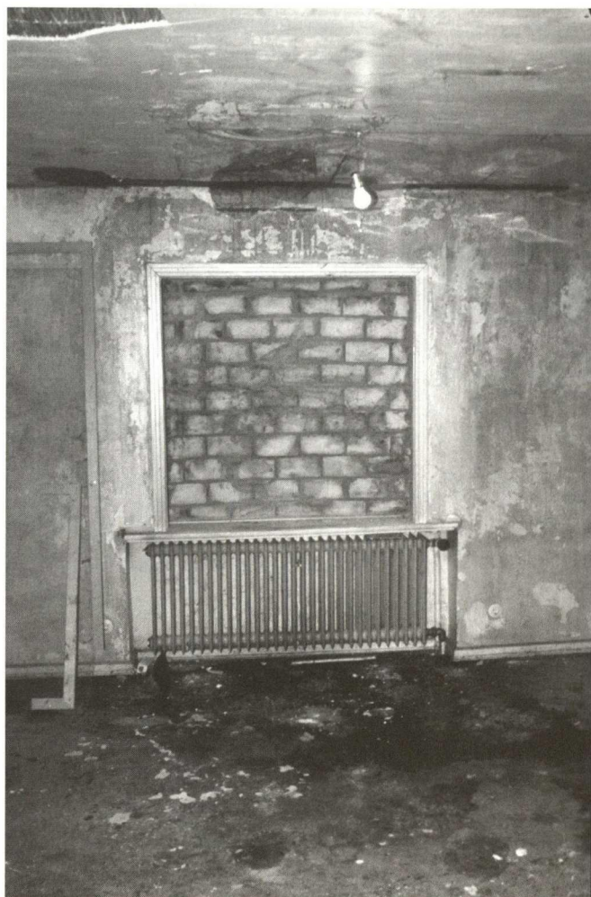
Situation before the demolition, room already cleared out, the frames removed (cf. Heritage at Risk 2002/2003, fig. on p. 97)
