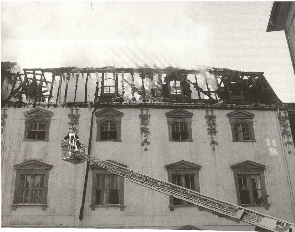
Weimar, Anna Amalia Library, west facade on the day after the fire (3 September 2004), smouldering fires not yet extinguished (photo: J. Seifert)
