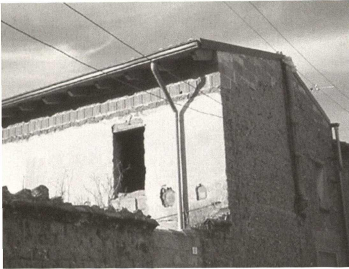
The top part of this earthen building shows repair with cement blocks (Terralba, Sardinia)
