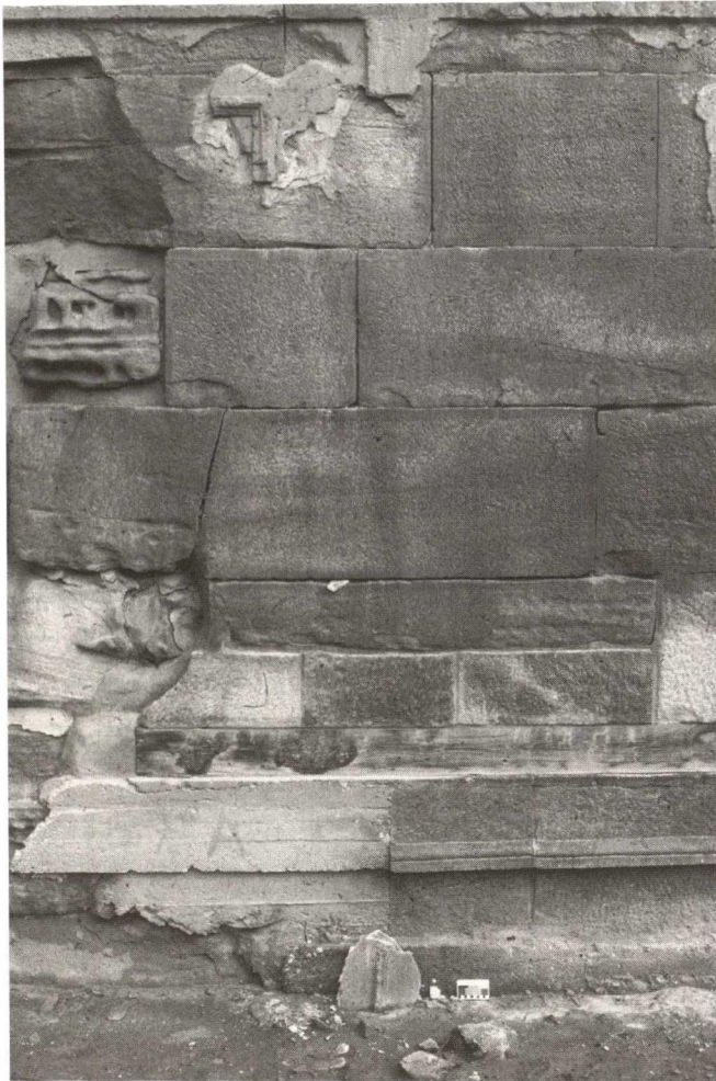
Qasr al Bint, condition of stucco decoration
