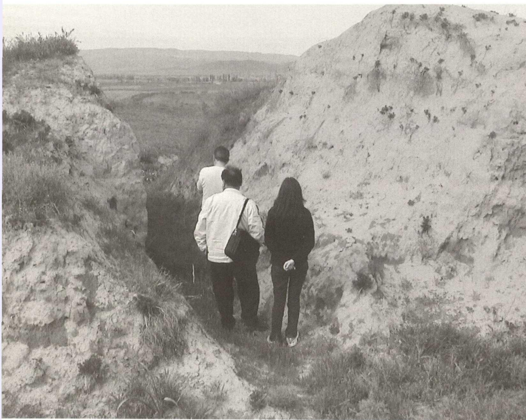
A part of the pradakshina patha with the highly threatened mudbrick structures of the cella (left) and the outer wall
