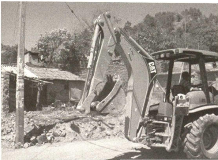
Destruction of adobe buildings in Hueyapan (Morelos)
