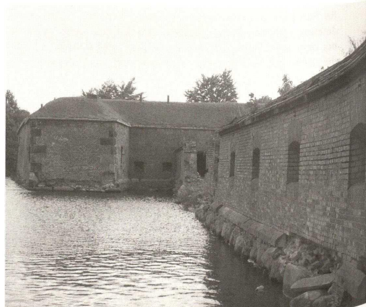
Vistulamouth Fortress in Gdansk, view on to the damages of the bastion's bricks caused by water
