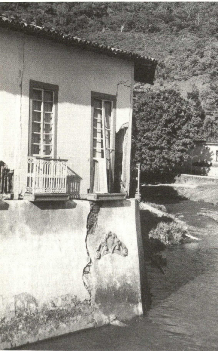
Building after flood damage
