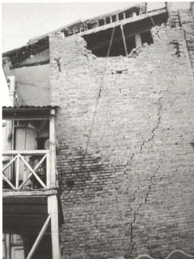
Earthquake damage in Tbilisi Historic district Residential house in Kvemo Kala micro-quarter after the earthquake
