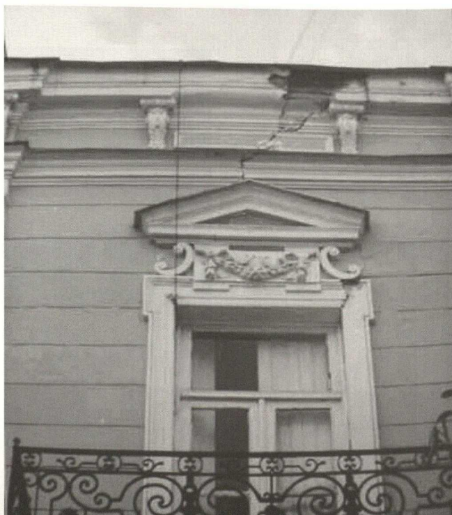
Parapet of a residential house (in Sololaki quarter) damaged by the earthquake
