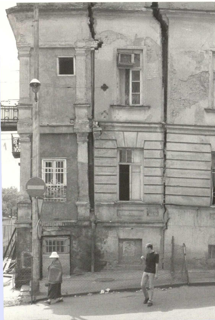
Residential house in Mtatsminad after the earthquake
